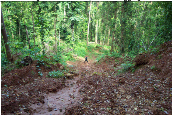
Plate 3 Erosion caused by no water bars.
