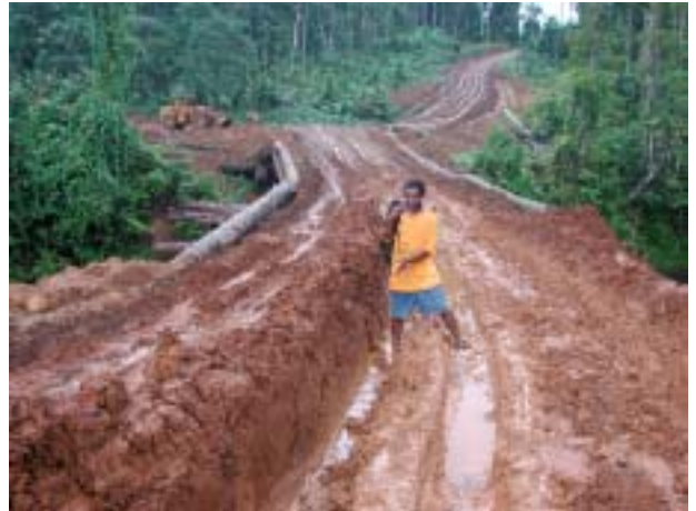
Figure 6. Poor drainage and deep ruts are a major problem on forest roads.
